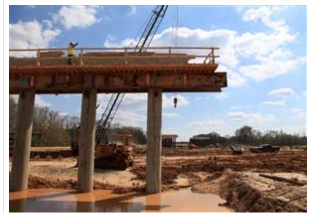
A crew from Hill Brothers Construction works on a bridge on the section of Tenn. 385 under construction between Tenn. 57 and Macon Road. Photo: Lance Murphey
